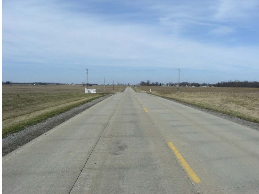
Figure 23. Section Illinois Highway 2, Cumberland County (2016) at 16 years age.
