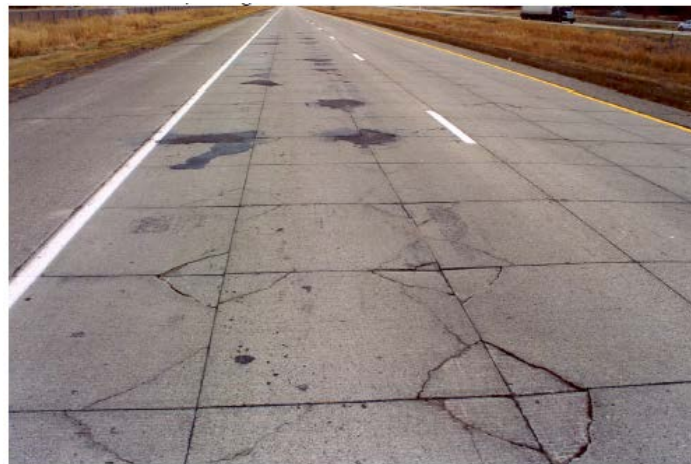
Figure 5. MnRoad test section with 4x4 ft joint spacing and corner fatigue cracking. (Burnham, 2005)
