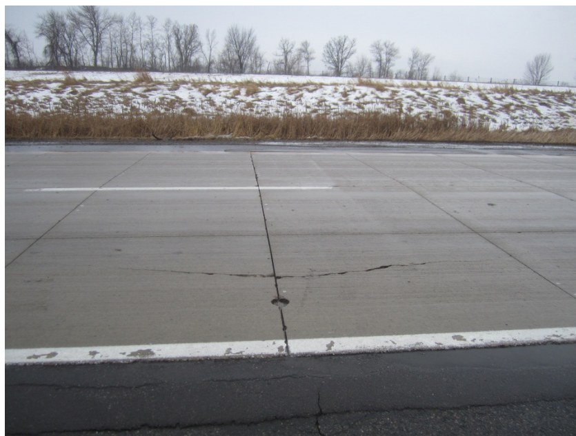
Figure 7. MnRoad section with 6x6 ft joint spacing and 6 inch PCC over AC exhibited predominantly longitudinal cracking (A few corner cracks occurred along outer edges).
