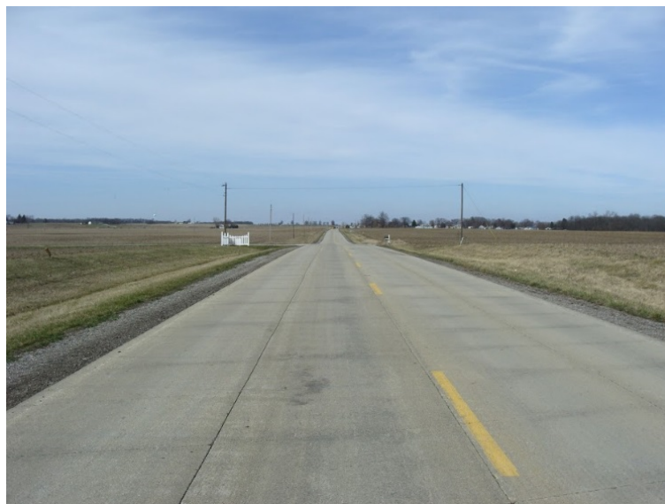
Figure 12. Photo of Illinois CH 2, zero cracking after 15 years, zero longitudinal cracking.
