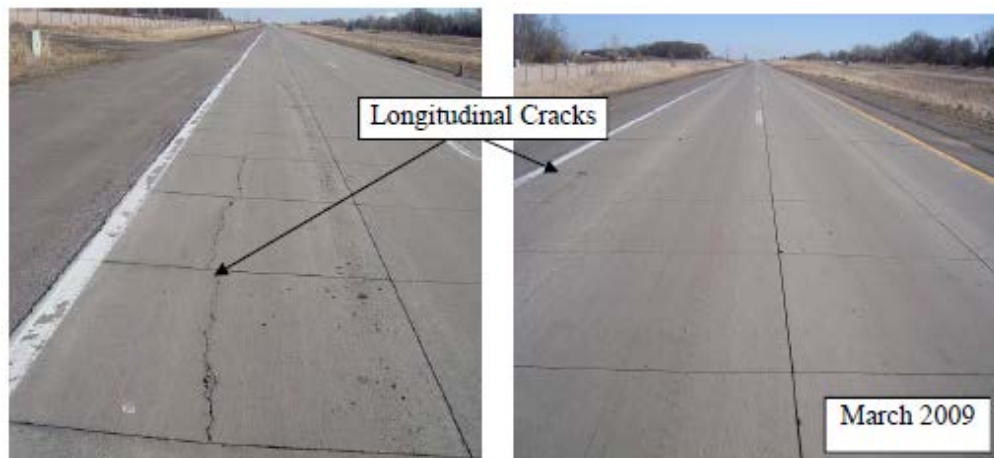
Figure 3. MnRoad SJPCP Test Sections with 6x6 ft joint spacing and longitudinal fatigue cracking. (Vandenbossche, Barman, Mu, Gatti, 2011)
