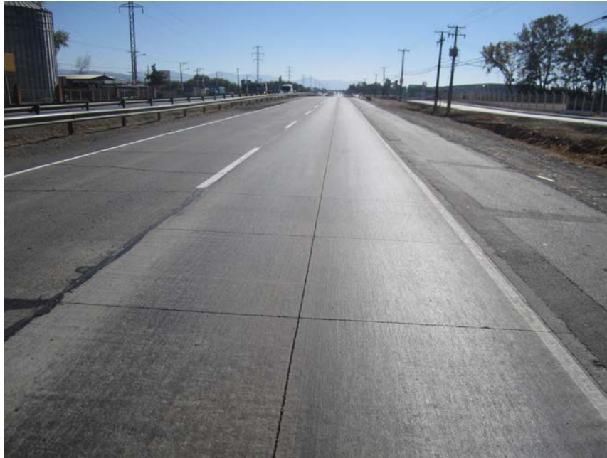
Figure 15. BCOA project (outer lane) on Route 5, the Pan American Highway that runs north/south in Chile carrying very heavy truck traffic Talca, Chile (6Wx6.7L ft joint spacing).
