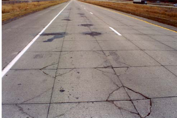
Figure 8. Cell 94 MnRoad driving lane with 3 in PCC, 4x4 ft joint spacing (longitudinal joints within wheelpaths, and 94 percent slabs with corner cracks. (Burnham, 2005)
